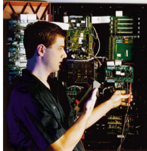
Our Technicians Are Factory-Trained to Maintain Complex Fire Alarm Equipment.
